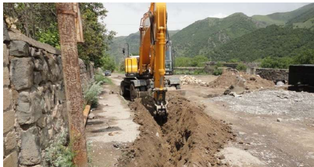
Construction of water infrastructure in the town of Kalbajar in the occupied Kalbajar district Source: www.armenianfund.org | 2013
